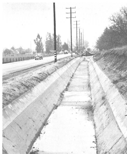
ge Canal, near Loma Linda, Calif., was lined in 1886 with 1 in. of cement mortar. Much of the original lining is still in good condition.
